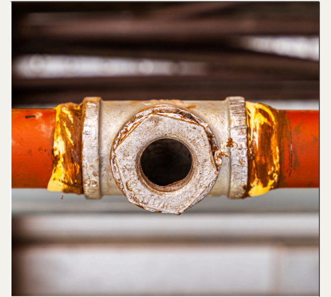
FIRE PUMP INSTALLATION
